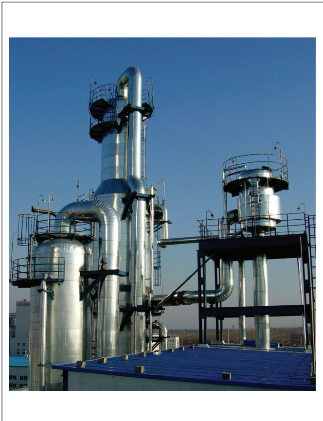
Figure 3. VB Multipressure distillation system
