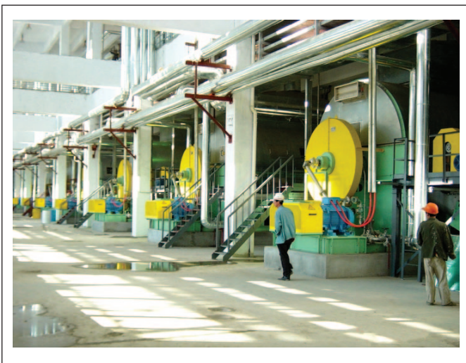
Figure 4 Steam tube drying units
